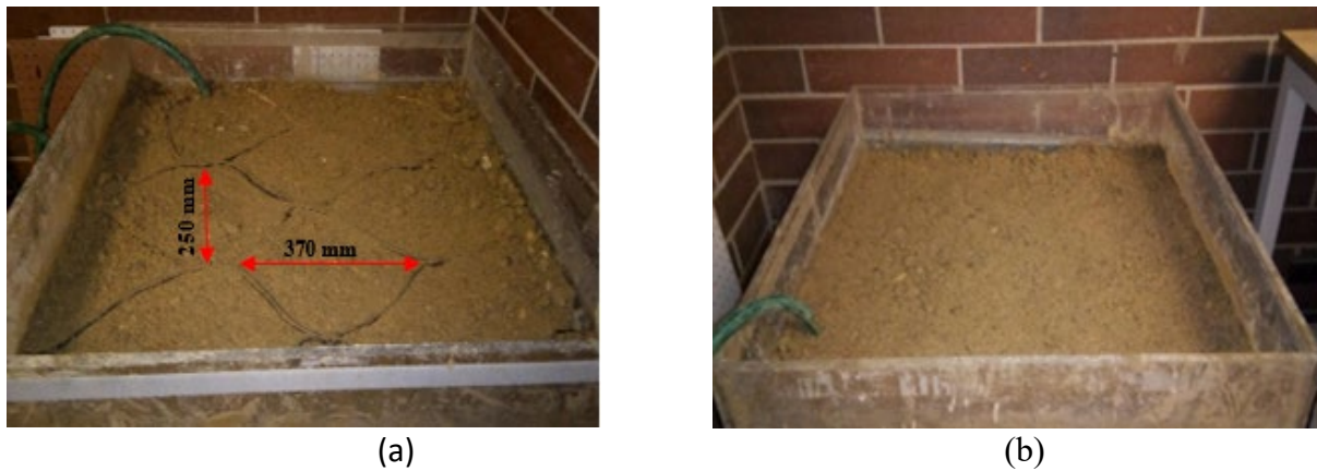
Figure 7. (a) Geocell placement in hybrid reinforced section and (b) Complete hybrid reinforced section after compaction.
