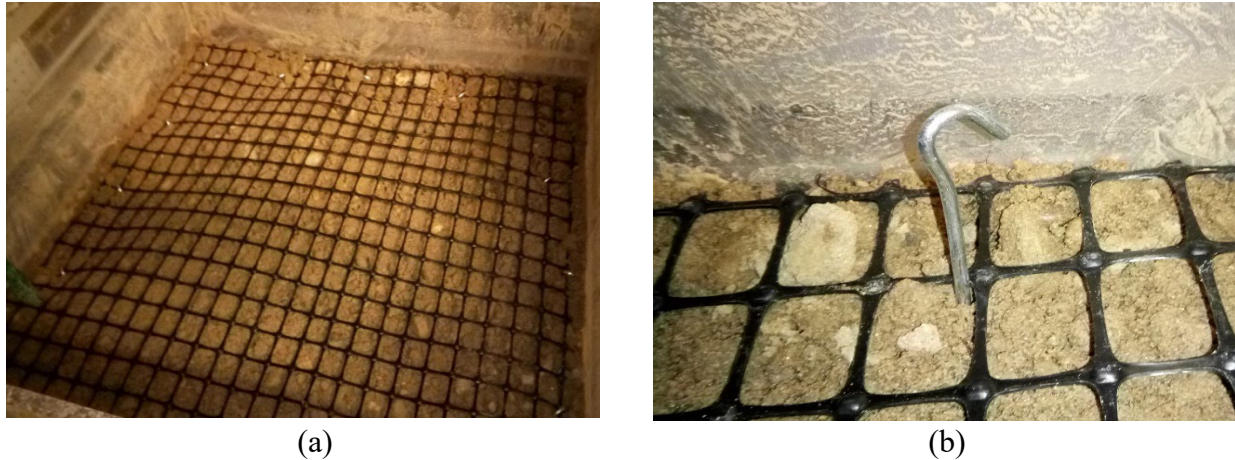
Figure 6. (a) Geogrid placement in hybrid test section and (b) Anchoring of geogrid using steel peg.
