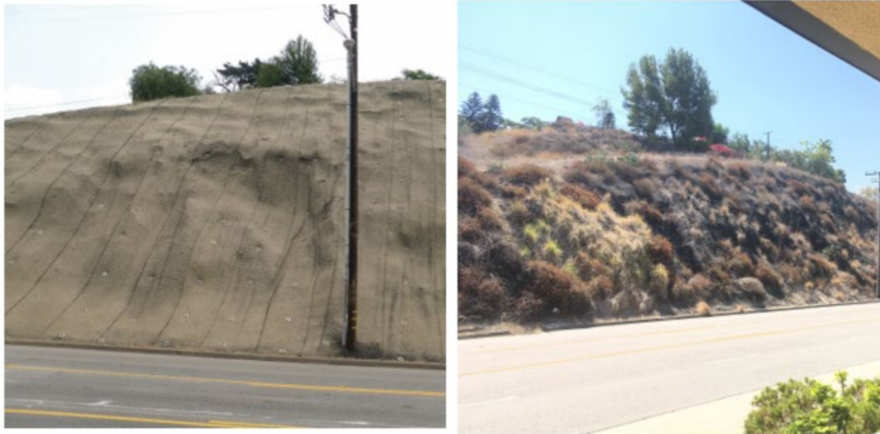
Figure 4. Soil Nailing system with geomat with DTWM reinforcement and hydromulch before and after the growth of vegetation.
