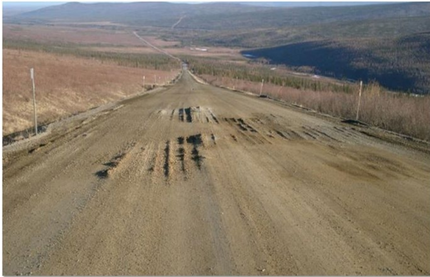
Figure 6. Moisture Induced Rutting.
