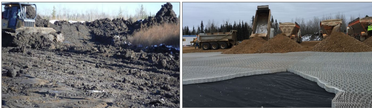
Figure 1: a) Existing soft soil subgrade and b) Partially stretched bottom layer NPA geocell
