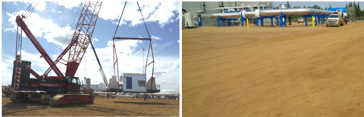
Figure 4: a) 275 tonne Crane lifting compressor on May 8, 2017 and b) Condition of pad after one and a half year of service on July 27, 2018 (Pictures courtesy Mr. Mark Bonnell, Program Manager, Strike Group)
